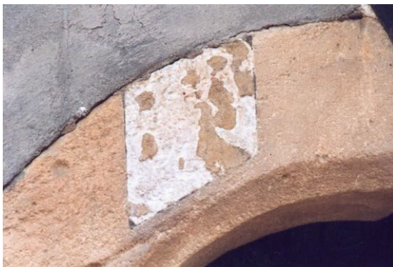
Fig. 2 The application of improper kind of sandstone
