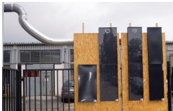
Fig. 6 Connection of collectors to the air-conditioning unit (Hovorka)
